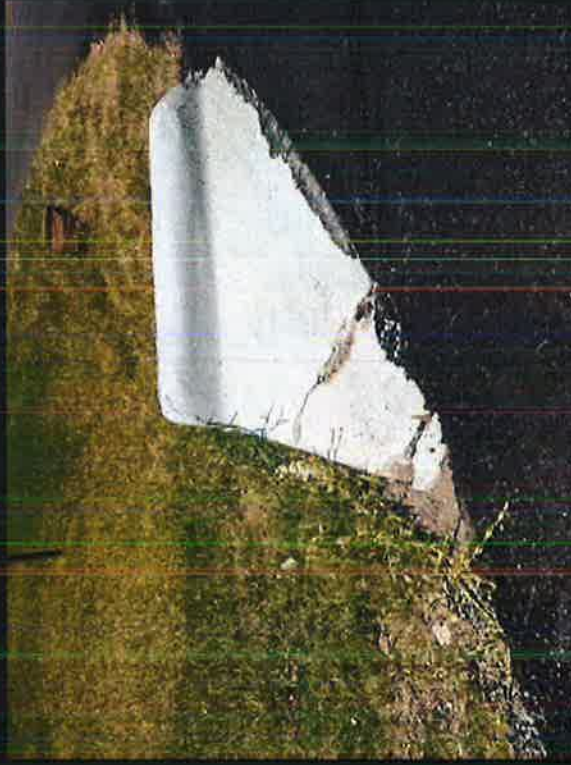
Culvert headwall crack sealed
