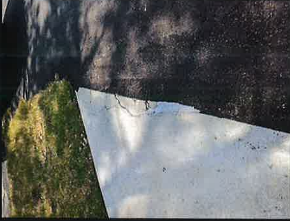
Culvert headwall crack sealed
